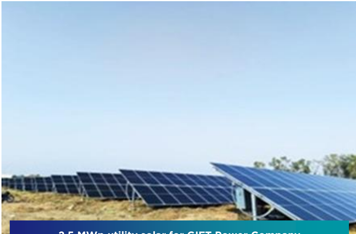
2.5 MWp utility solar for GIFT Power Company
