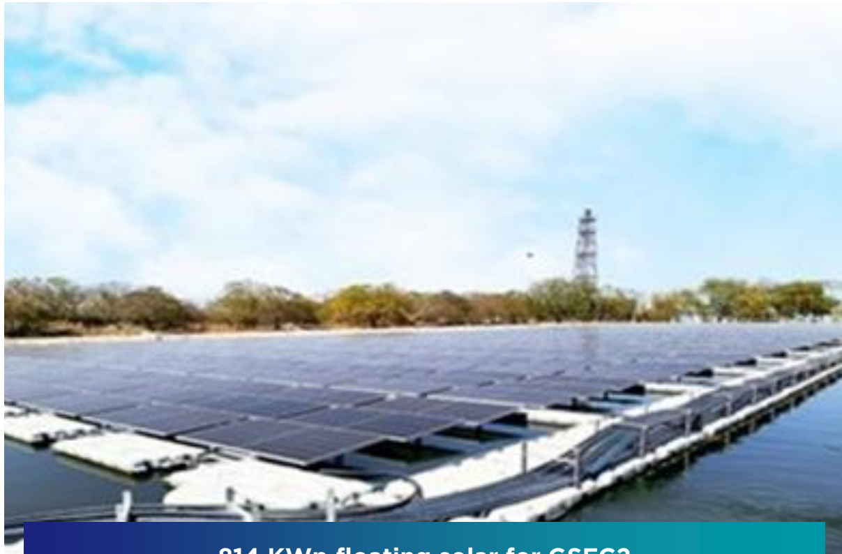
814 KWp floating solar for GSFC2
