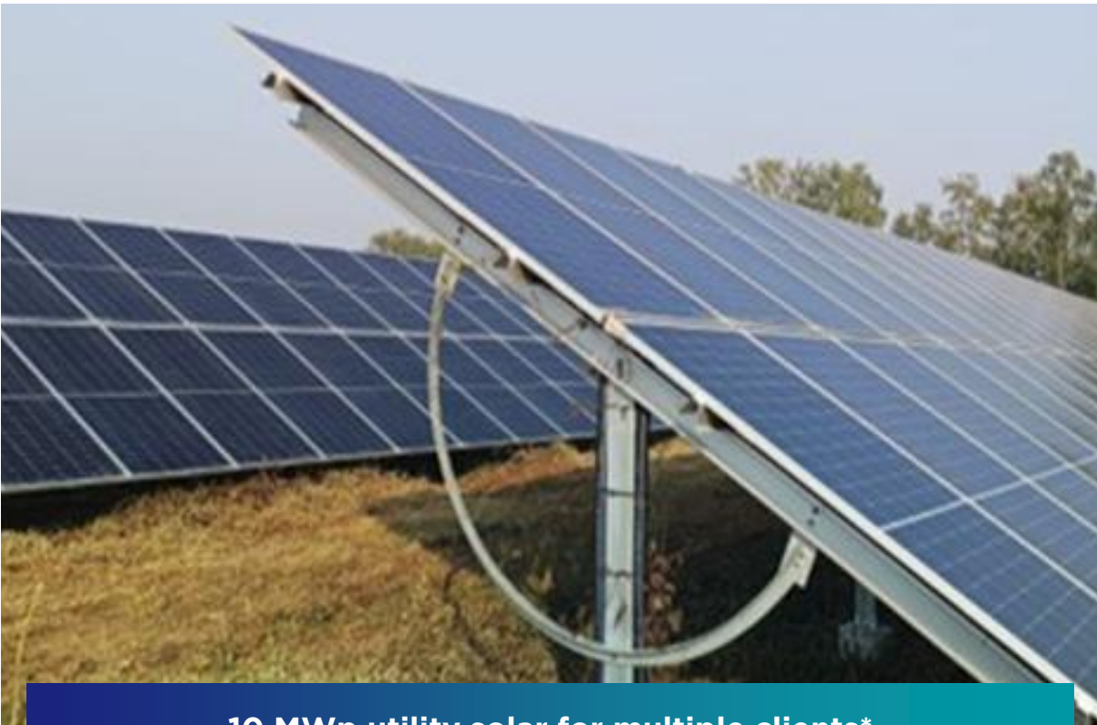
10 MWp utility solar for multiple clients*
