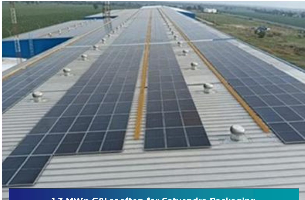
1.3 MWp C&I rooftop for Satyendra Packaging
